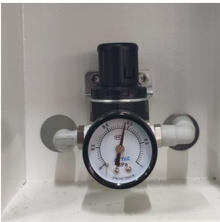
Fig F- Feeder air pressure value pressure 0.55MP
