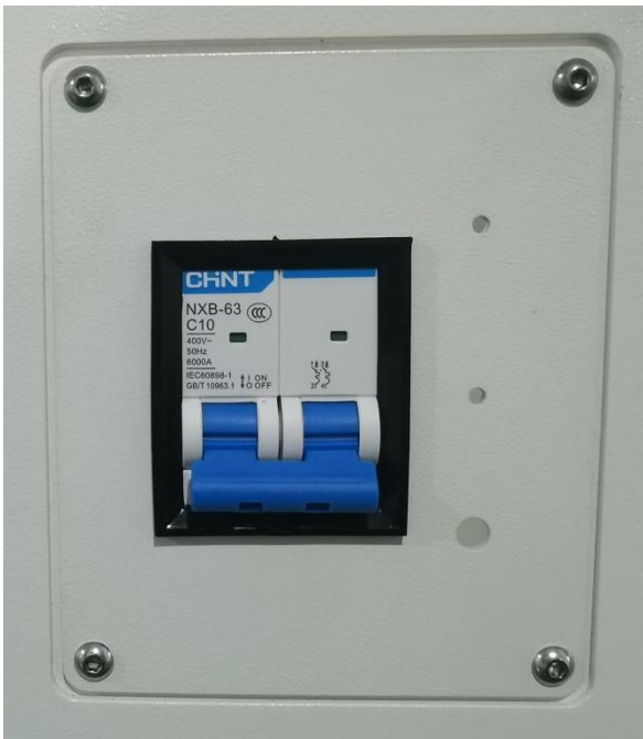
Fig G- Air switch
